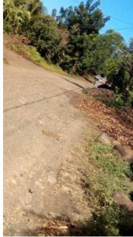
Figure 5. But you see the picture, the road is in bad condition, it's in bad shape. You cannot use the bicycle, because with roads in this condition, such as this one, it makes bicycling a lot more difficult... Yeah of course, they ride the bicycle, but they have to go really slow because they cannot go fast, because if they go fast there could be an accident. Captured by Participant 8, 2018.
